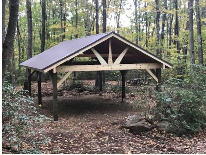
Pavilion constructed in Roger Sherman campsite for use of Wilderness Patrol during summer camp. (Photo courtesy of Ranger Dave)
