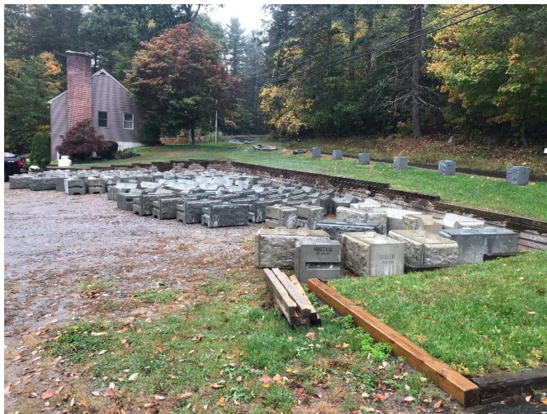
Retaining wall blocks sitting in camp parking lot awaiting installation at the Bogan Waterfront
